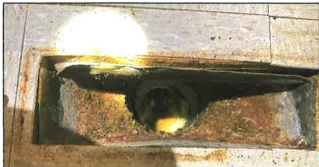
Flaking corrosion extends down boot into metal duct elbow...note corrosion at bottom duct elbow
