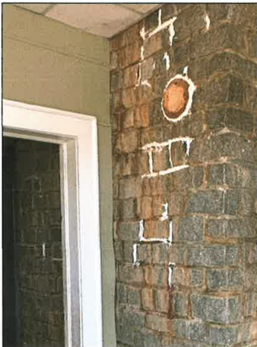
Apparent attempts to mitigate leaks around chimney
