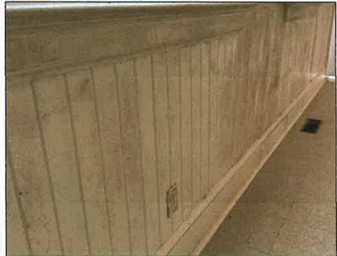
An example of the pervasiveness of mold in this building (below). Wall outlet plate corrosion is apparent source of air infiltration
