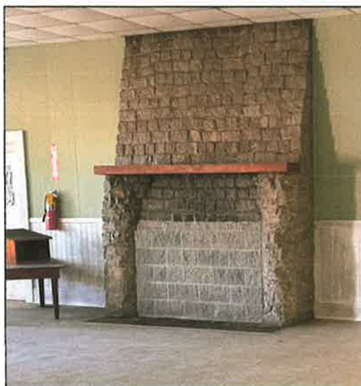
Both Chimney Fireboxes blocked up Note mold on wainscoting both sides of Chimney
