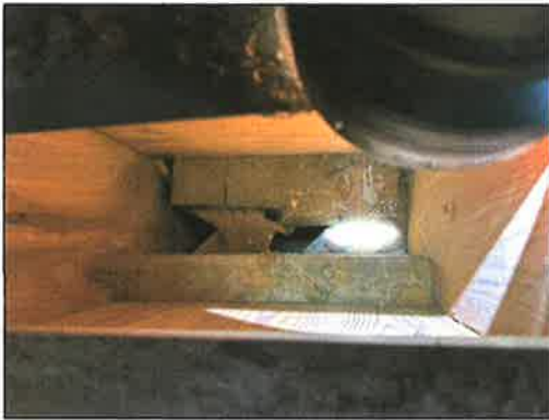
Wall gap in front of Air Return plenum: Note floor sheathing (top of photo) projecting into wall cavity (center of photo)
