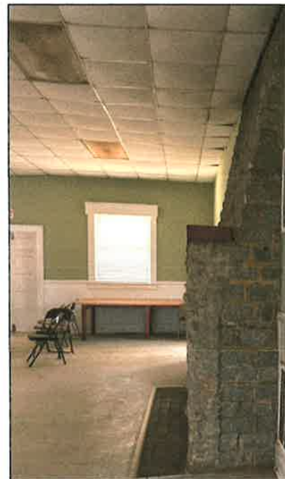
Cupped ceiling tile, above , stained light fixtures, staining on chimney surface from roof leaks
