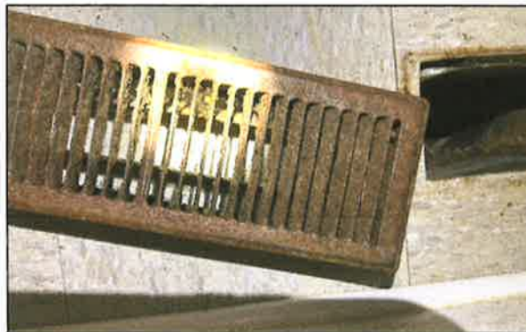
Typical surface corrosion on metal floor registers
