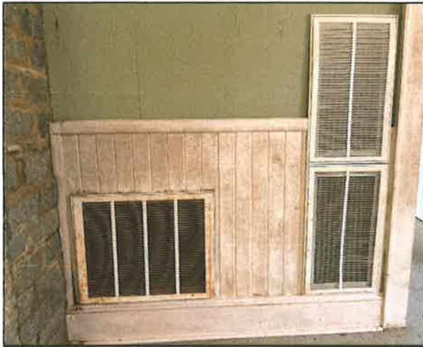
Corroded return grill, extensive mold development around air returns; mold spores pulled into air handling unit and conveyed throughout entire building
