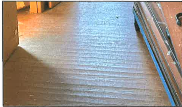
Cupped hardwood flooring on east wing
