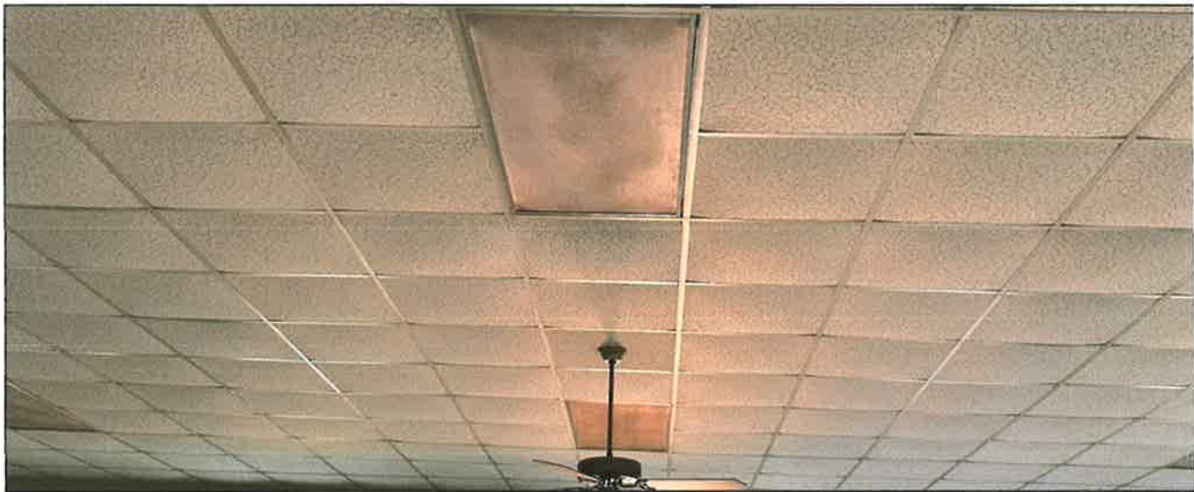
In meeting hall, cupped 2'x2' ceiling tile (with fiberglass insulation batts on top). Condition is; frequently indicative of elevated humidity in building
